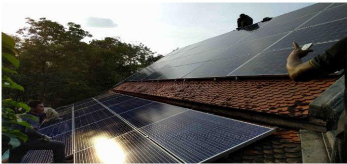
New solar panels at Wongsanit Ashram, Thailand
